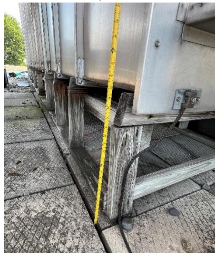
Photo 17: Light-frame dunnage appearing unsecured to the roof metal deck or structural framing.
