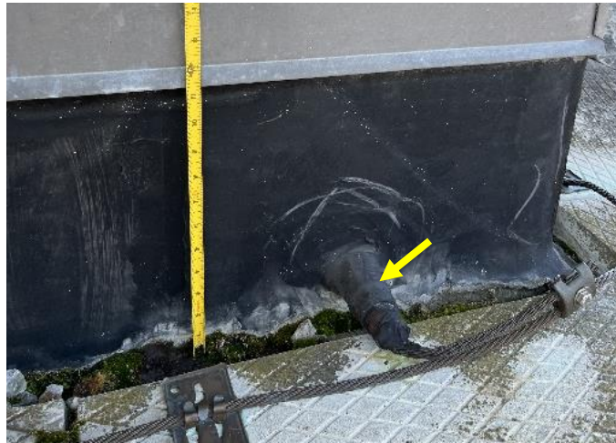
Photo 11: Low lightning cable wall penetration (arrow).
