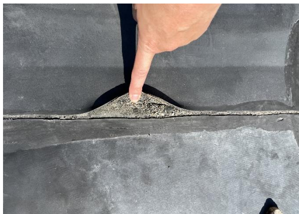
Photo 20: Edge of EPDM membrane seam is partially unadhered.
