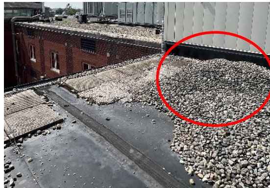
Photo 8: Areas with a high concentration of stone ballast (circled) and adjacent area with no ballast.
