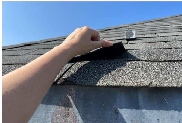
Photo 25: Unadhered corner of asphalt shingle.
