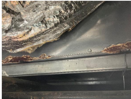
Photo 4: Staining and corrosion on metal duct above ceiling in an area of stained ceiling tiles.
