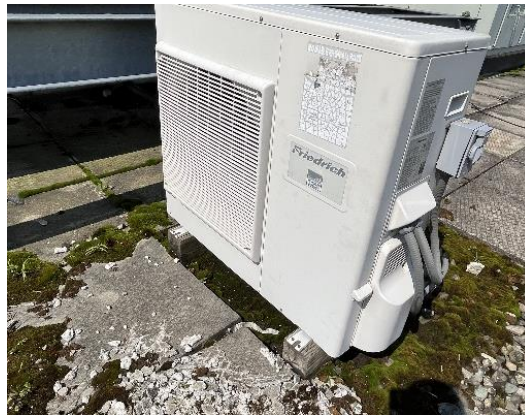
Photo 13: Rooftop equipment supported on wood sleepers above the roofing membrane.
