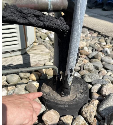
Photo 10: Cracked sealant at a few sealant-filled flashing pockets.
