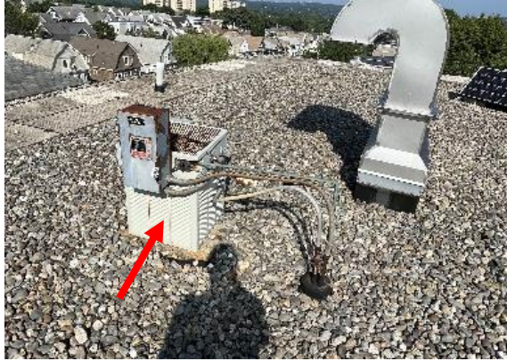
Photo 18: Unsecured rooftop equipment at the mechanical mezzanine roof.
