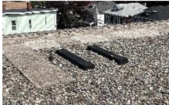
Photo 16: Abandoned rooftop equipment curbs and capped conduit penetration.
