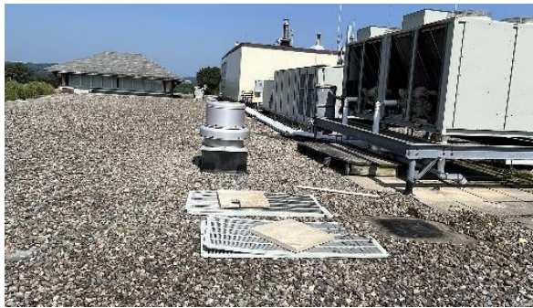
Photo 19: Loose metal grilles on the main roof, held down with precast concrete pavers.
