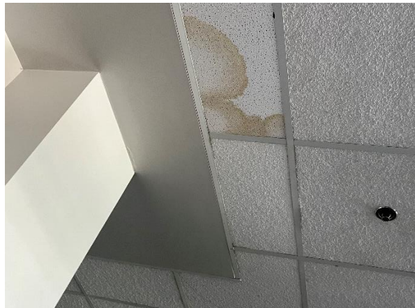
Photo 2: Stained ceiling tile below roof.
