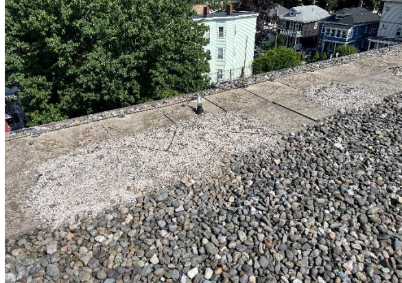
Photo 7: Deteriorated precast concrete pavers at the perimeter of the main roof.
