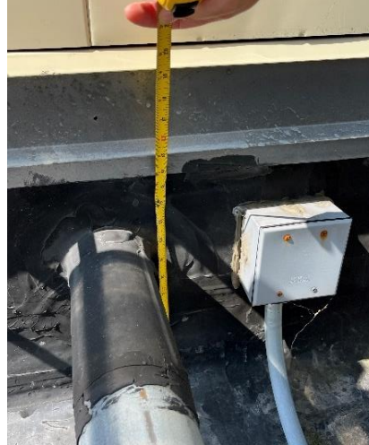
Photo 15: Low electrical conduits and pipes.
