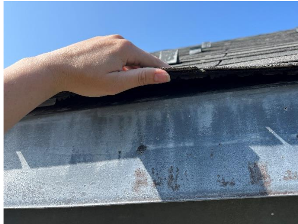
Photo 24: The bottom of the lowest course of shingles is not adhered to the metal flashing.
