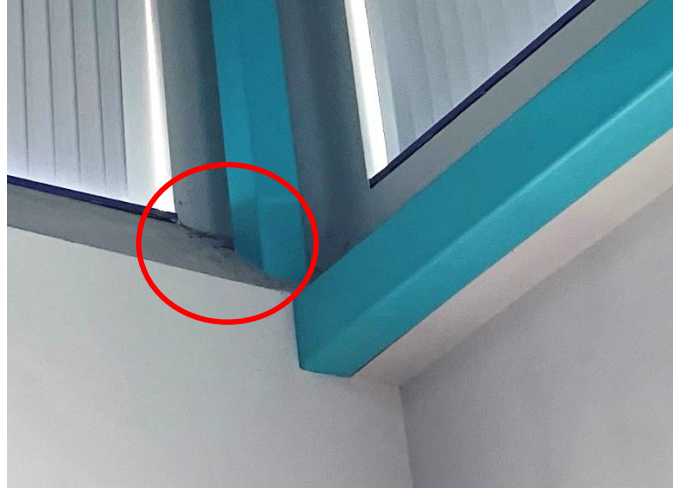
Photo 6: Potential damaged interior finishes at corners below clerestory windows at hipped roofs (circled).
